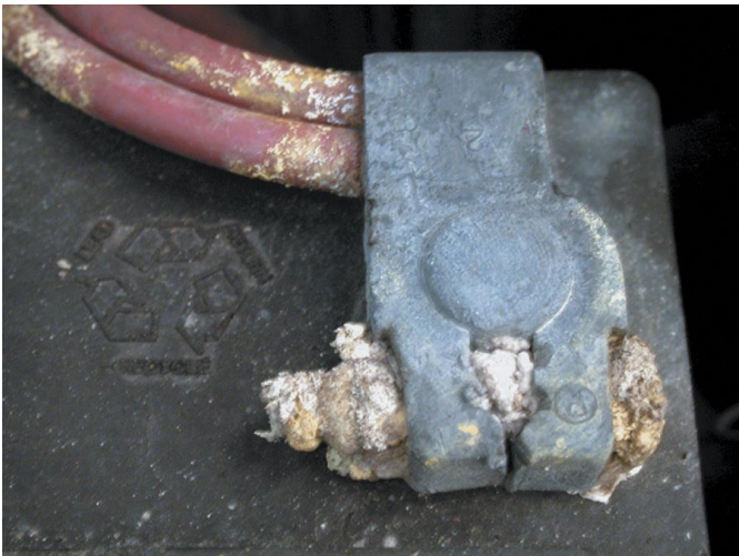
Figure 18. Corroded cable connections can cause slow cranking.
