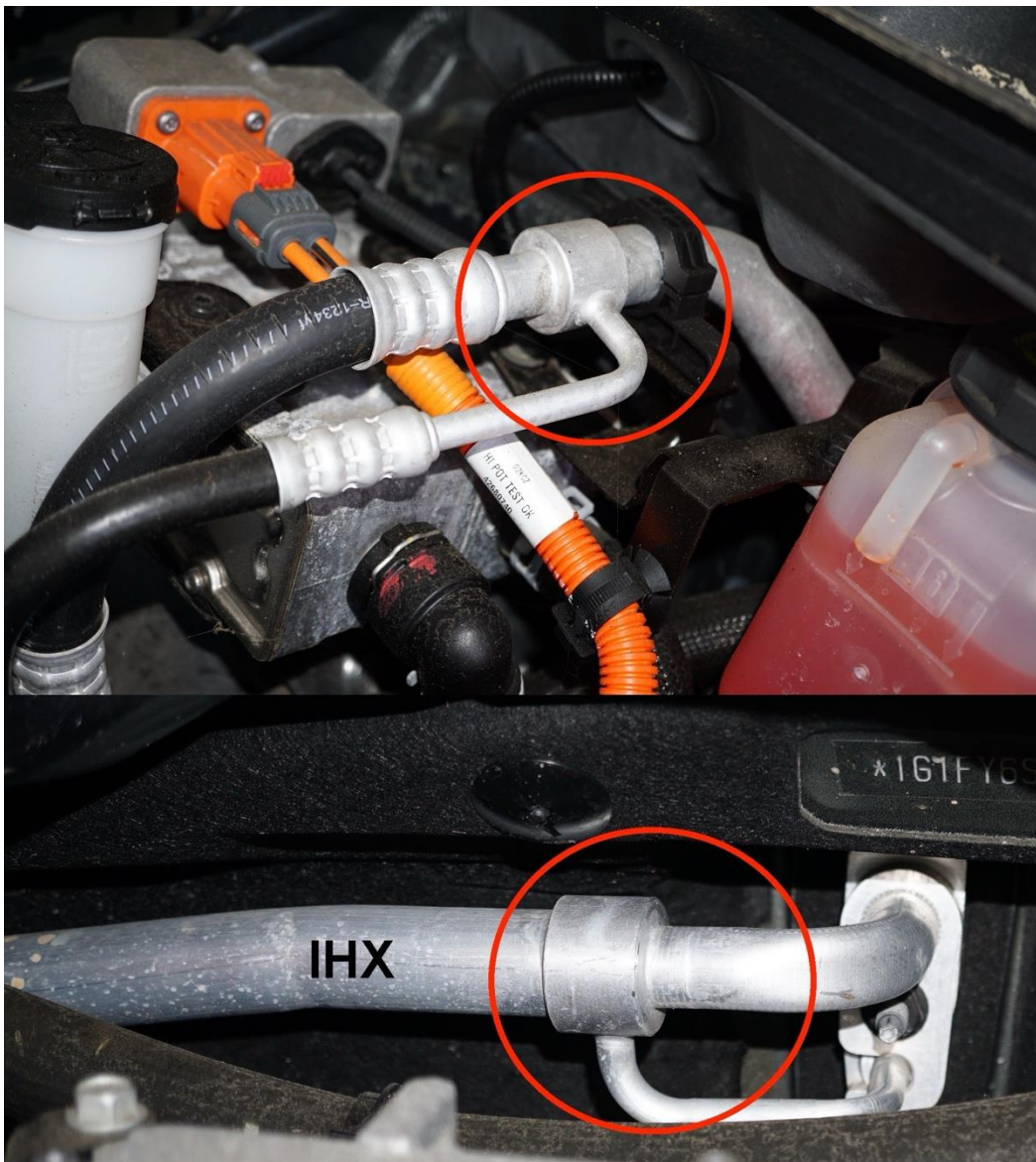
Figure 37. An internal heat exchanger (IHX) is recognized by the combined refrigerant lines (circled).
