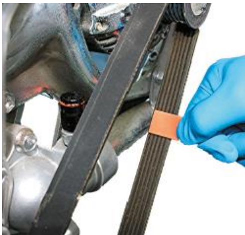
Figure 11. A belt wear gauge should fit tightly into the belt grooves. A loose fit means the belt is worn and should be replaced.
