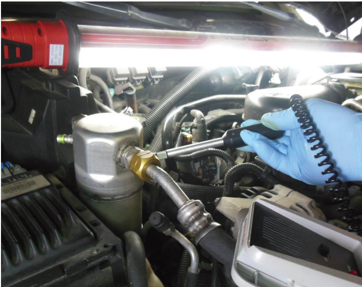
Figure 16. An electronic leak detector being used to locate a possible leak in a system. For best results, move the detector probe completely around each fitting and connection.
