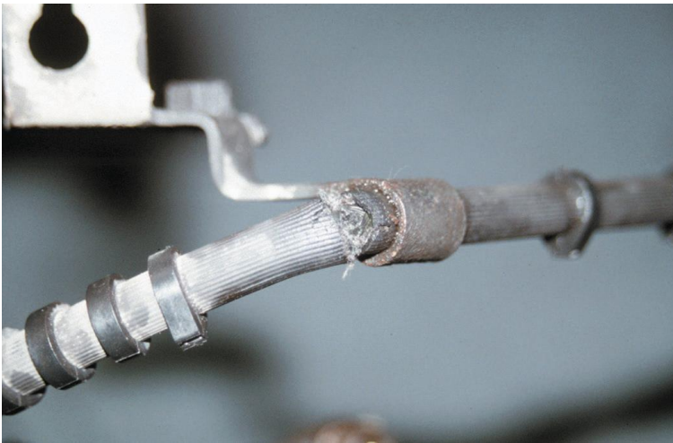
Figure 16. This brake hose should be replaced.
