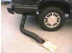
FIGURE 6.6 Always connect an exhaust hose to the tailpipe of the engine of a vehicle to be run inside a building.
