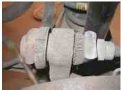
FIGURE 49.17 Check all rubber bushings for excessive cracking.
