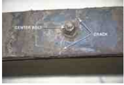
FIGURE 49.21 The center bolt is used to hold the leaves of the leaf spring together. However, the hole for the center bolt also weakens the leaf spring. The crack shown is what a technician discovered when the leaf spring was removed during the diagnosis of a sagging rear suspension.
