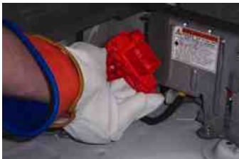
FIGURE 43.5 The service plug on a Toyota Prius, which is located in the trunk and is orange in color. Toyota recommends that the technician wear high-voltage gloves when removing the disconnect plug.
