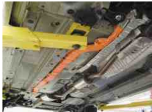
FIGURE 43.8 The high-voltage wiring on this Honda hybrid is colored orange for easy identification.
