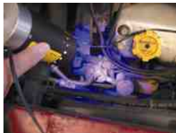
FIGURE 38.8 A black light being used to look for refrigerant leakage after a fluorescent dye was installed in the system.
