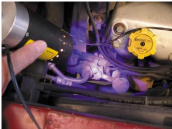
FIGURE 13-9 A black light being used to look for refrigerant leakage after a fluorescent dye was installed in the system.
