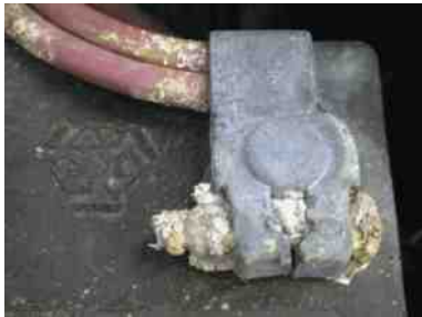
FIGURE 18-2 Corrosion on a battery cable could be an indication that the battery itself is either being overcharged or is sulfated, creating a lot of gassing of the electrolyte.
