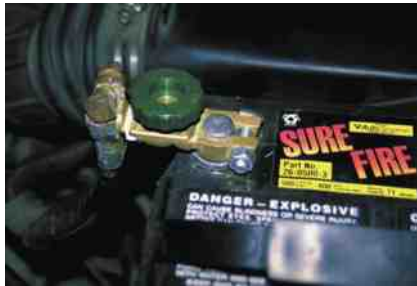
FIGURE 18-17 After connecting the shut-off tool, start the engine and operate all accessories. Stop the engine and turn off everything. Connect the ammeter across the shut-off switch in parallel. Wait 20 minutes. This time allows all electronic circuits to “time out” or shut down. Open the switch—all current now will flow through the ammeter. A reading greater than specified (usually greater than 50 mA, or 0.05 A) indicates a problem that should be corrected.
