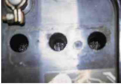
FIGURE 18-1 A visual inspection on this battery shows the electrolyte level was below the plates in all cells.
