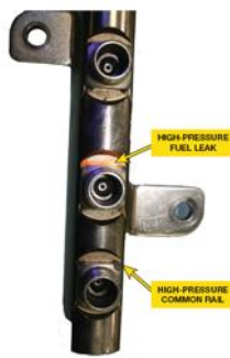
FIGURE 13–23 Using a black light, fluorescent dye is visible at the location of high-pressure fuel leak.
