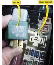
FIGURE 8-49 A typical relay showing the schematic of the wiring in the relay.
