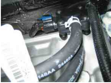
FIGURE 4-19 A differential pressure sensor showing the two hoses from the diesel exhaust particulate filter.
