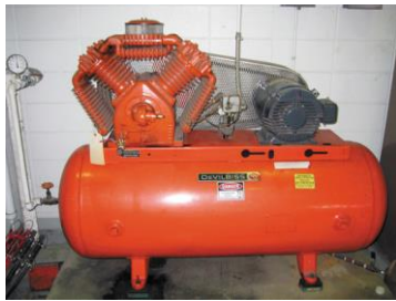
FIGURE 5-1 A typical shop compressor. It is usually placed out of the way, yet accessible to provide for maintenance to the unit.
