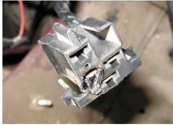
FIGURE 35-1 A partially melted electrical connector indicates that excessive current flow was present. The cause of the excessive current should be located and corrected before the engine is started.
